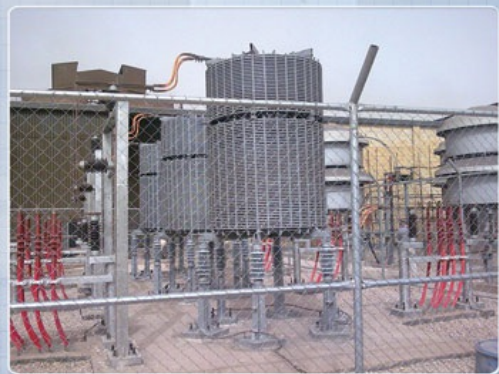
4mH/2000A/50KA Are furnace Series Reactors Ahvaz - KSC
